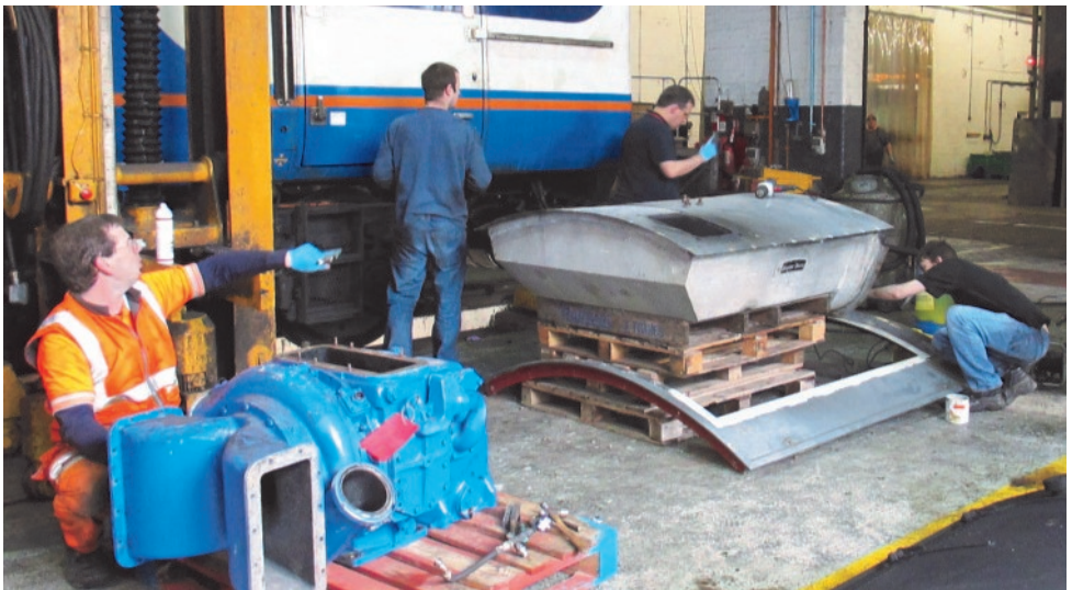
Opposite: With the engine room roof off, Steve helps guide the silencer off 41001. 04/04/15 © James Trebinski Above: All systems go! Everyone at work either on the silencer or turbo. 04/04/15 © Alex Wood
